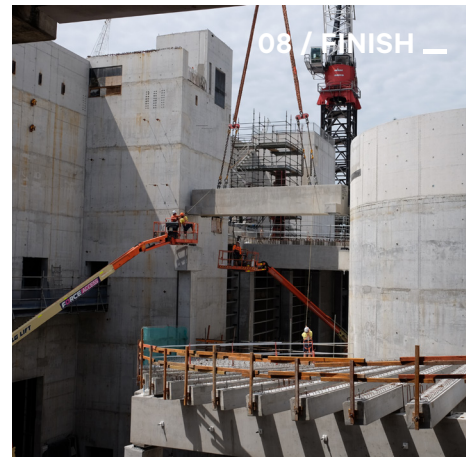
Our solution allowed Lendlease to maintain their original program, despite the pressure of design changes throughout the project. By completion, 100 critical lifts for elements weighing between 10 and 100 tonnes had been made without incident.
