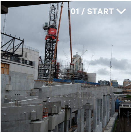
A congested inner urban construction site surrounded by light rail, public roadways, existing buildings, additional construction work and the general public posed a number of challenges.
