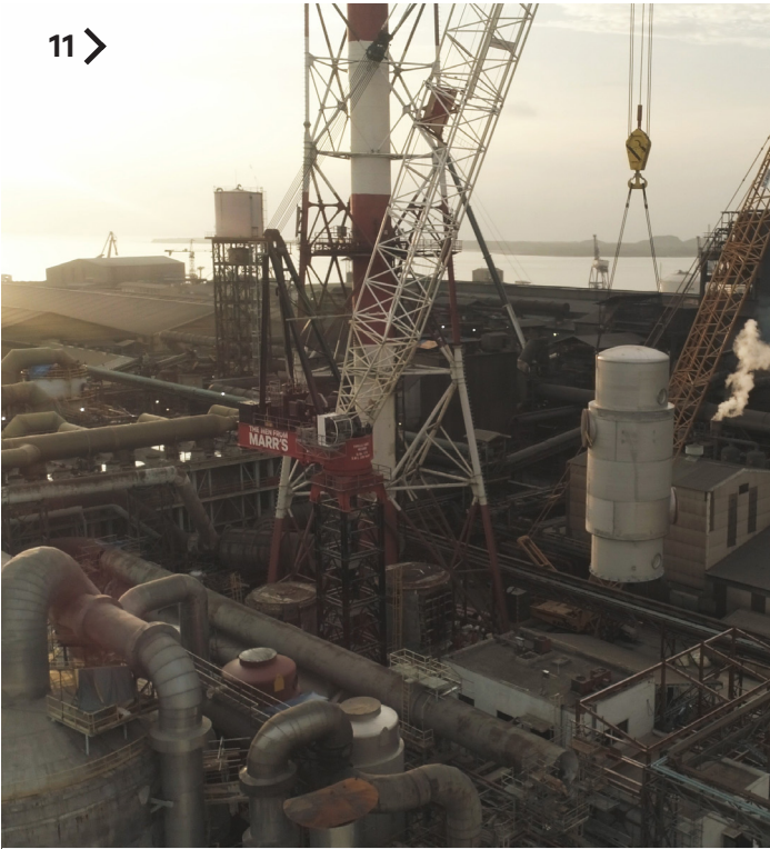
After the old vessels were removed, new replacement vessels were installed using the same crane configuration.
