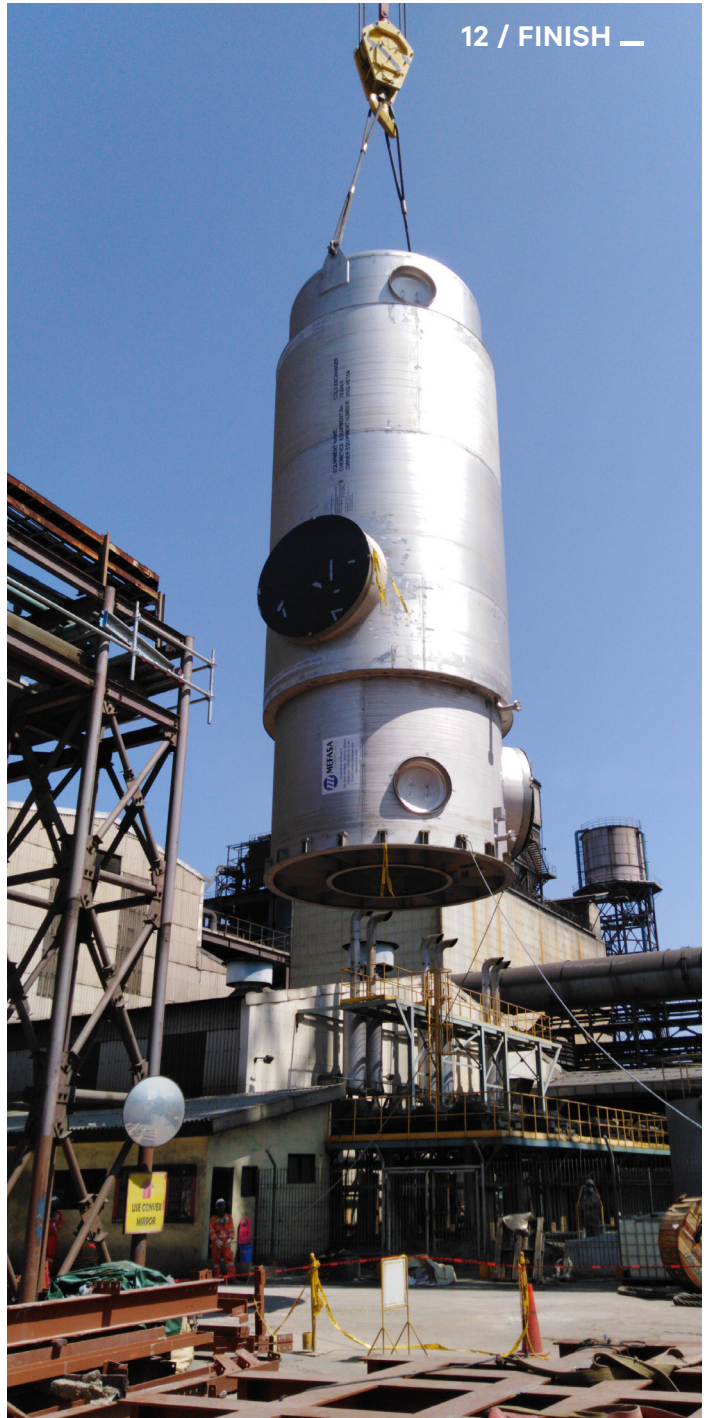
The last replacement vessel was installed with the 12-week scheduled shutdown resulting in the project being completed with less lifting, reduced risk to plant operations and a substantial cost benefit over the original planned methodology.
