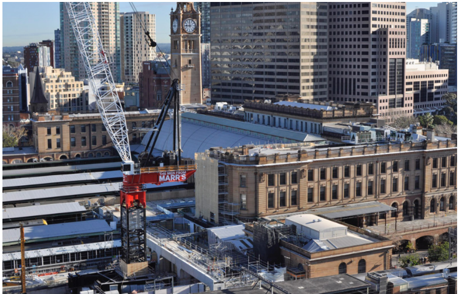
Marr's M1680D HLL was installed at Central Station to complete heavy lift and general construction requirements on above and below ground works associated with the redevelopment of Australia's busiest railway station.
